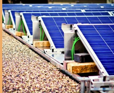
651 Harwood, Ajax, ON Size: 599 kW DC
