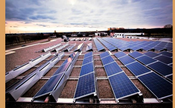
120 Van Kirk, Brampton, ON Size: 450 kW DC
